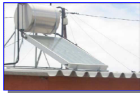
Solar water heaters
