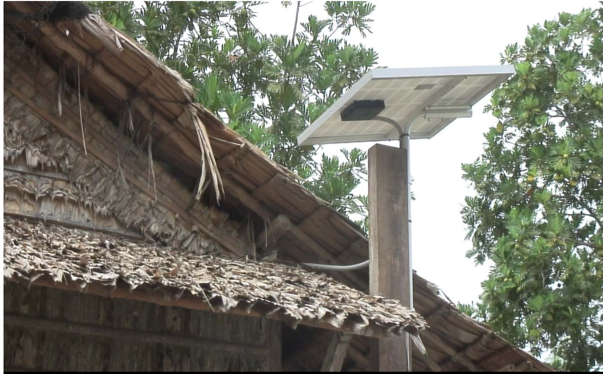
Solar Home Systems
