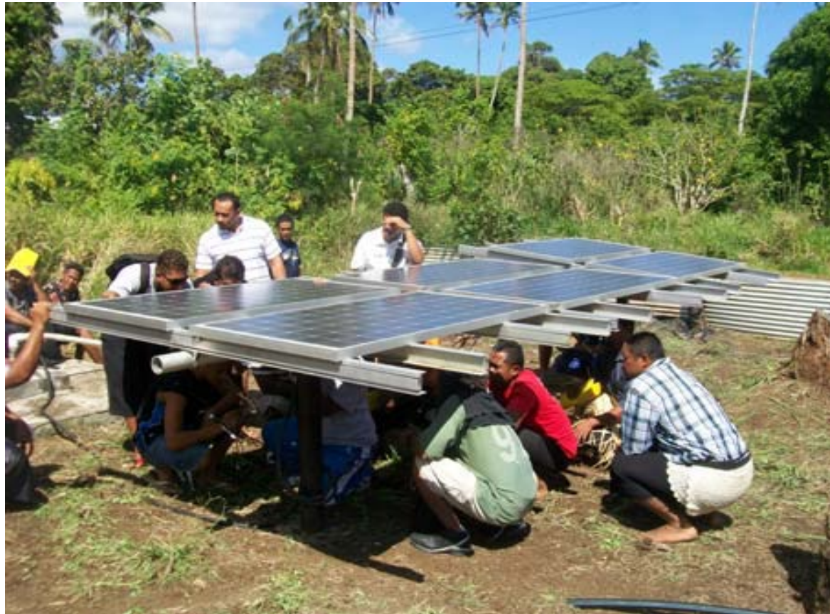
Solar powered water pumping system
