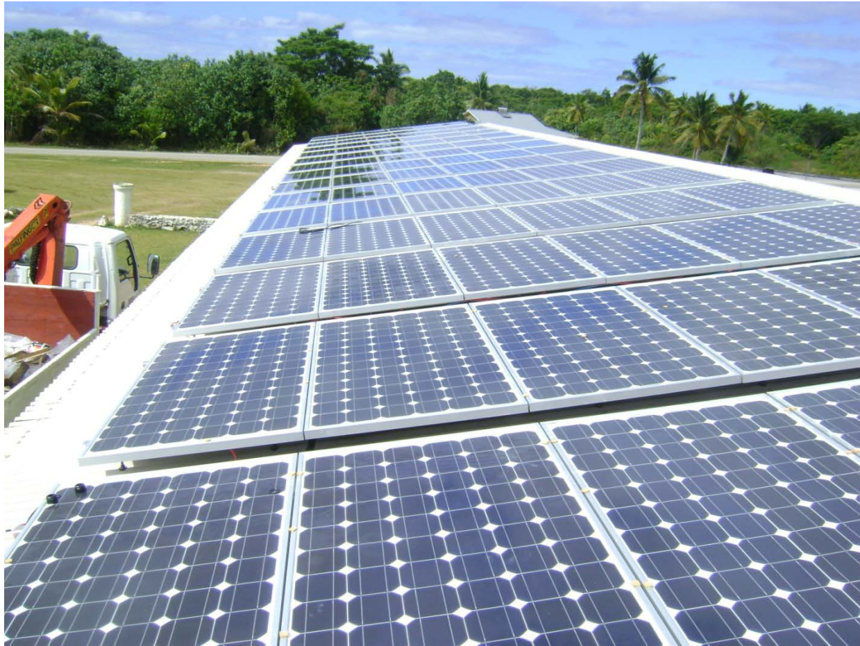
Grid connected Solar PV system
