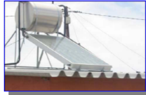
Solar water heaters
